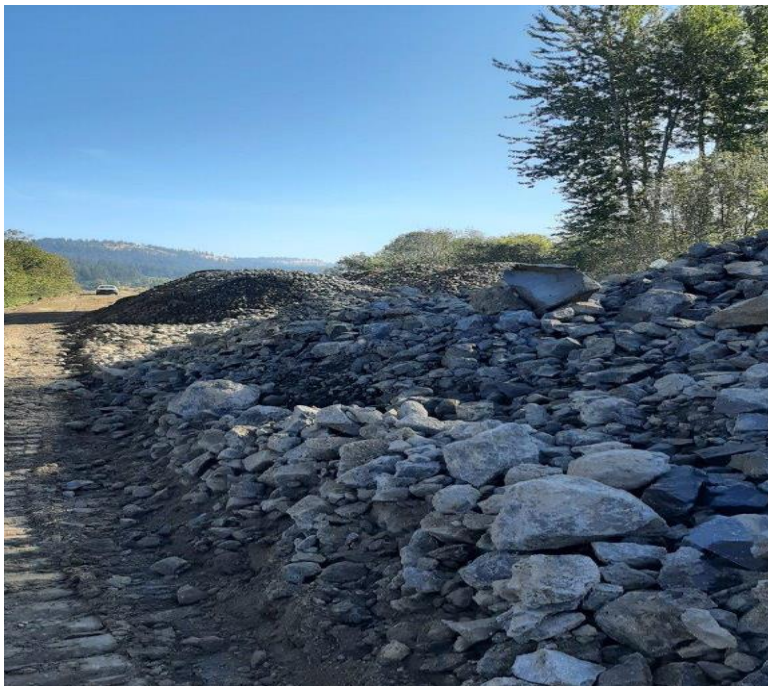
Photo 2. Structural fill is being stockpiled on top of the regraded levee on the east side of the breach in preparation for construction, which is scheduled for 2023.
