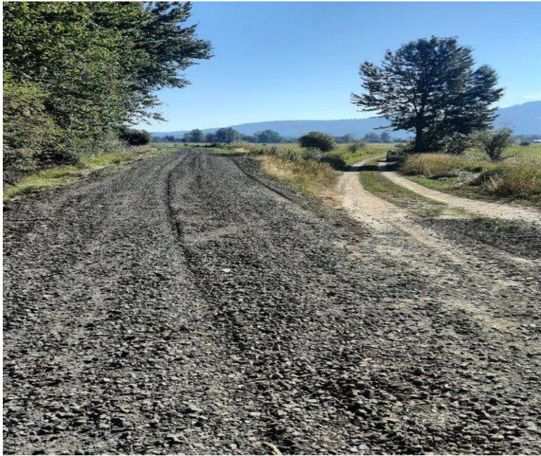
Photo 1. The construction access road across the top of the levee (left) has been improved to provide dust abatement during dry weather conditions and to extend site access during variable weather.
