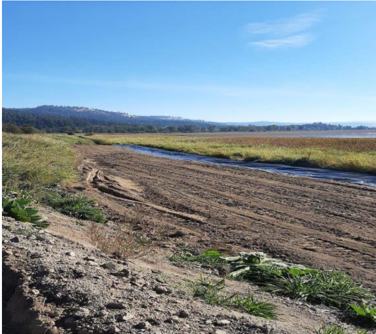
Photo 3. A low lying stockpile/staging area has been prepared adjacent to the levee breach and will be able to accommodate up to 2,000 CY of structural fill.
